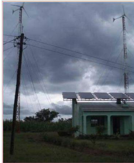
An image two of the 4kW wind turbines and solar panels at Elunyen community, Mzimba District
