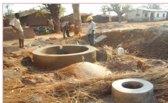
The image above shows the construction of a fixed dome biogas plant in Salima
