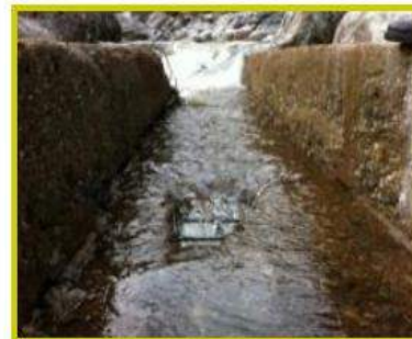
Smashed canal due to storm damage
