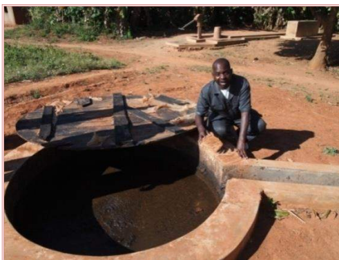
An image showing the ground opening of an outflow chamber filled with spent slurry (slurry that has been digested)
